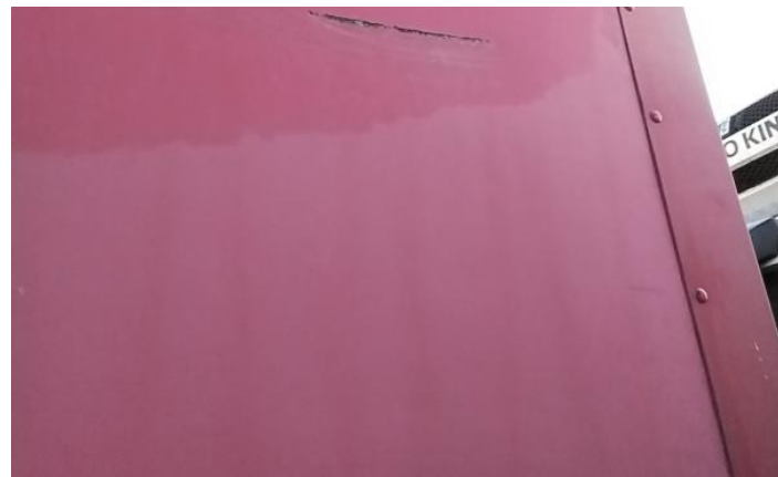
3: Door nsf Scratched Over 25mm Thru Paint
